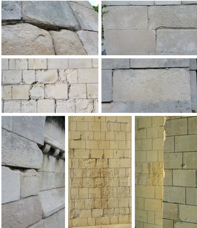
Figure 42: Photographs I took showing erosion and weathering of the stonework on Norwich Castle
